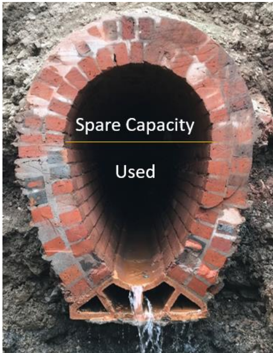
Figure 15 - Brick Lined Sewer with the concept of Spare Capacity- Image courtesy of St John Archaeology
